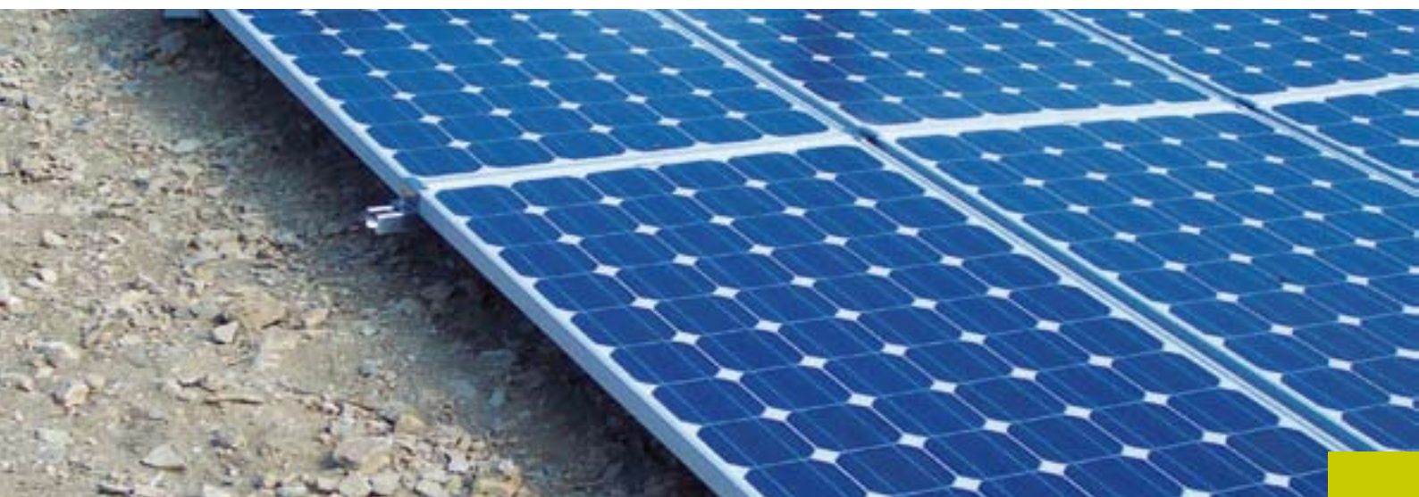
non integrato o a terra/not building-integrated or on the ground
